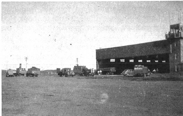
Truck loading during Penhold hangar demolition for the construction of the Parochial Centre, 1948
