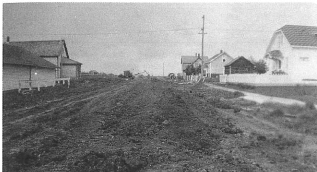
1949 Back-hoe ditching for re-installation of sewer and water line on 50 street (between 50th street and 51 avenue). Revelstoke Hardware on the left with "snorting-bar" to tie horses. North of hardware is the old St. Emile school used as a Youth Club. Across the road is the residence of Philippe Mercier, Armand Fauteux, Arthur Dufresne and Gédéon Demers
